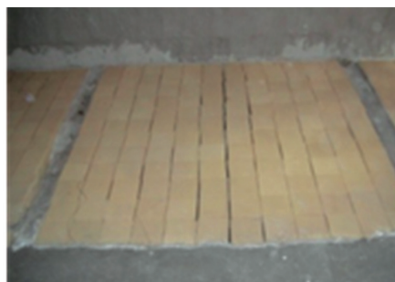
The old ceramic media had broken down and needed removal.
